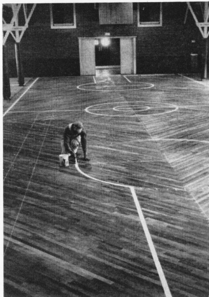
Here's the new surface of the floor in the SERA Center getting its finishing touches. It'll be fine for games and smooth for dancing.
